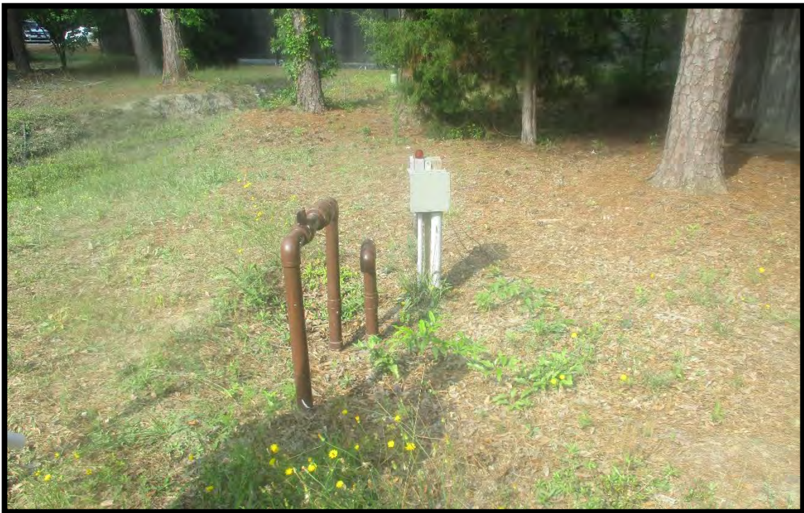
Photo #6 – There is a sewer lift station on the property. It wasn't clear who the pump station belongs to.
