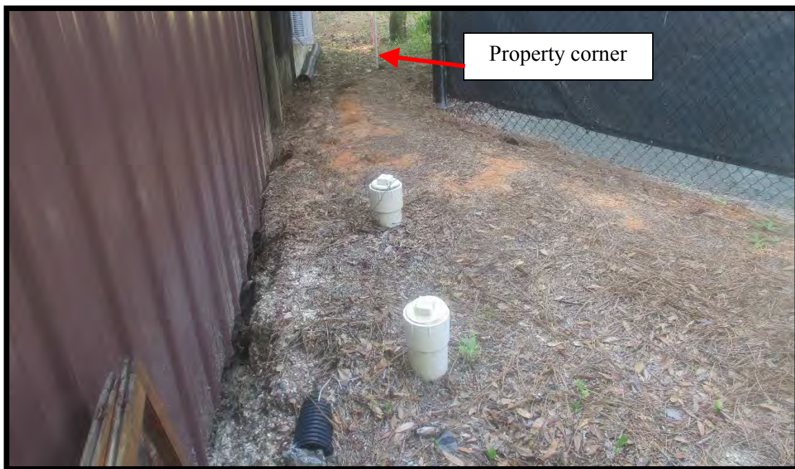
Photo #4 - This the rear of the building. The tennis courts were placed right up to the property line and the grade is raised 1-2 feet above the finished floor.
