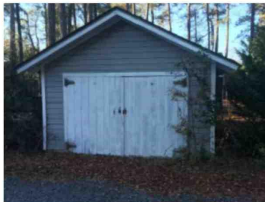
Opening to be secured. Color and material to match existing
