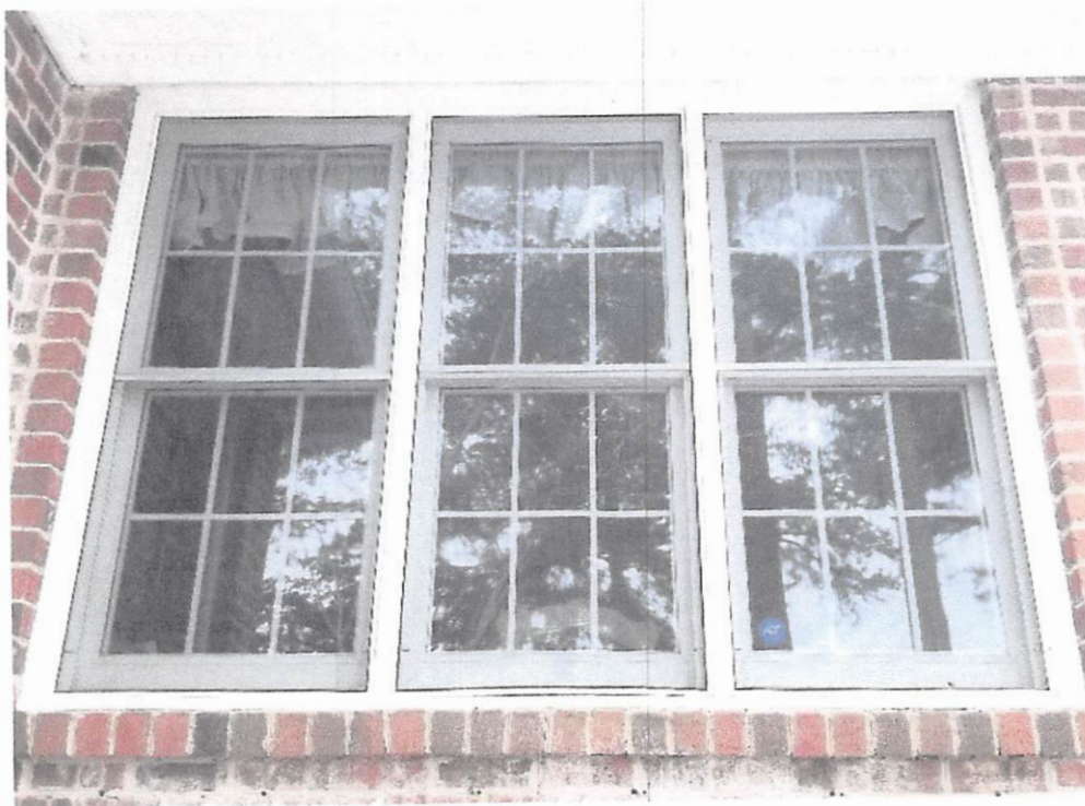
Exterior view of my kitchen windows. Please note the gap at the bottom of the middle window where insects crawl in.
