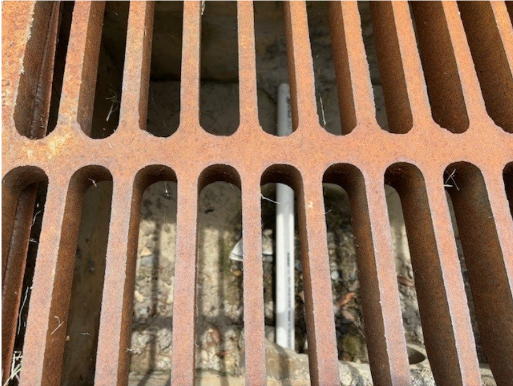
Photo 6 – Unknown PVC pipe through storm box on Backspin Lane
