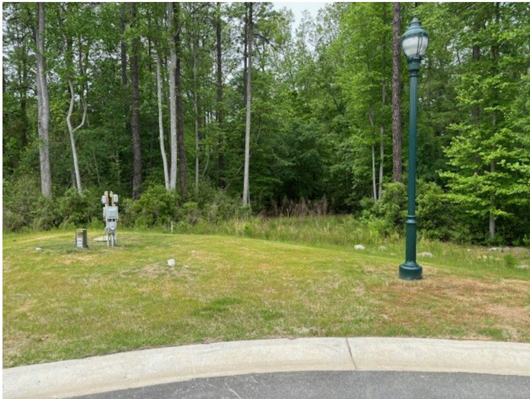
Photo 3 –Typical Grinder Pump Station and Street Light
