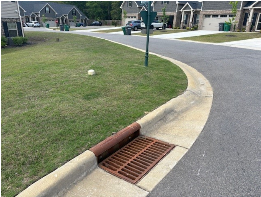
Photo 4 – Typical Curb Inlet Stormwater Box
