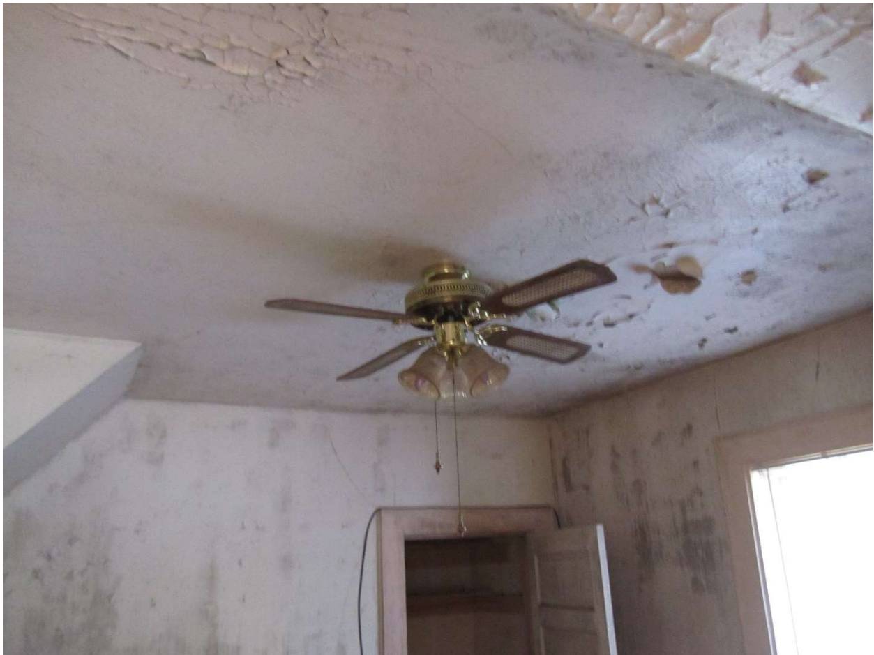
2 nd floor apartment #4 Mold and mildew, peeling paint
