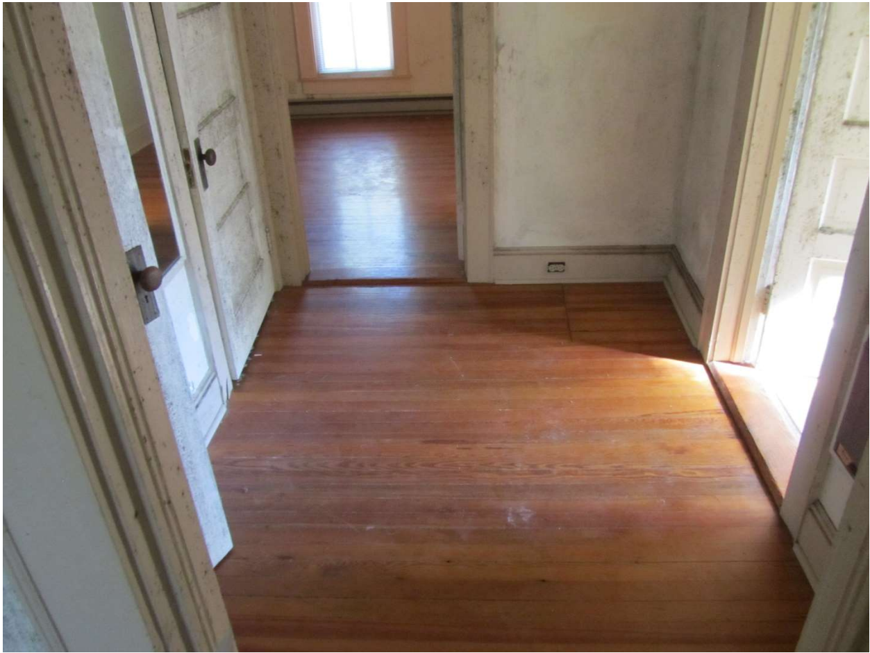
2 nd floor apartment #4 Heart pine flooring, mold and mildew
