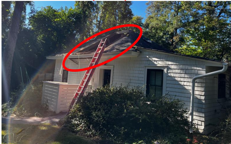
Picture K: Picture of the damage structure of the guest house in red:
