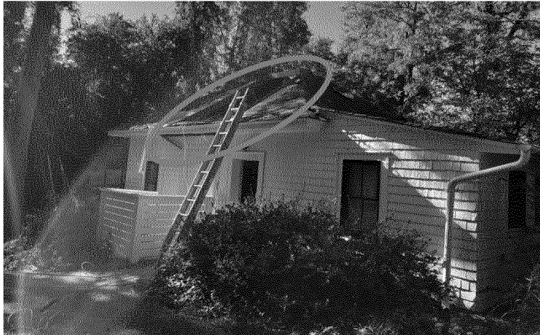
Picture K: Picture of the damage structure of the guest house in red:
